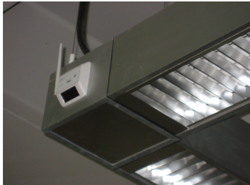
Wireless daylight sensors have been installed on light fixtures in perimeter zones. Image: UCSC.
